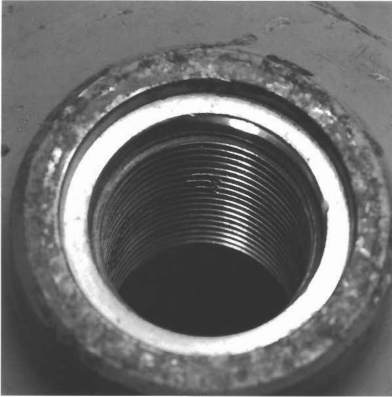
PHOTO 5. Damaged threads. This damage is easily seen with the naked eye, but the thread area is dirty and first needs cleaning (see NOTE 9), before proceeding with the visual inspection of the thread area.
