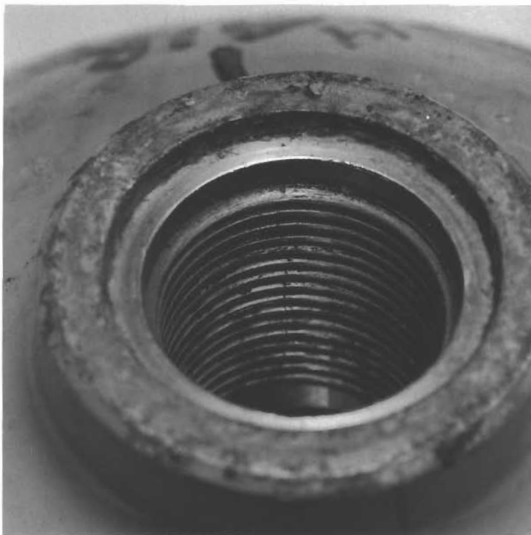
PHOTO 9. A crack easily seen with the naked eye, near the top or O-ring gland. A quick cleaning should be done, enough to verify that it is a crack.
